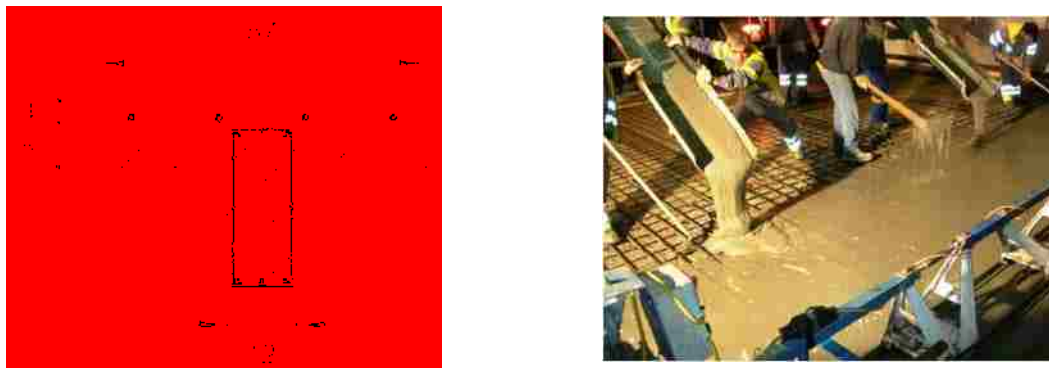
Figure 2-6 Cross section (dimensions in cm) with UHPFRC layer (in grey) and view of UHPFRC casting performed (Bruhwiler and Denarie, 2008)
